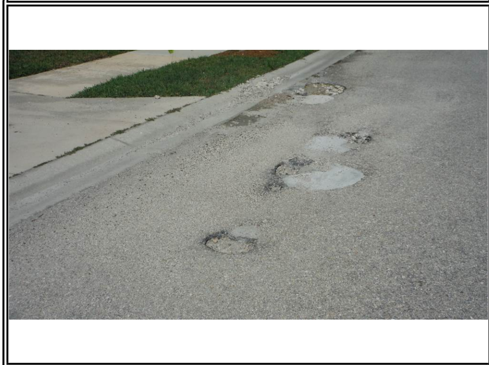
Photo No. 12 Isolated Potholes
