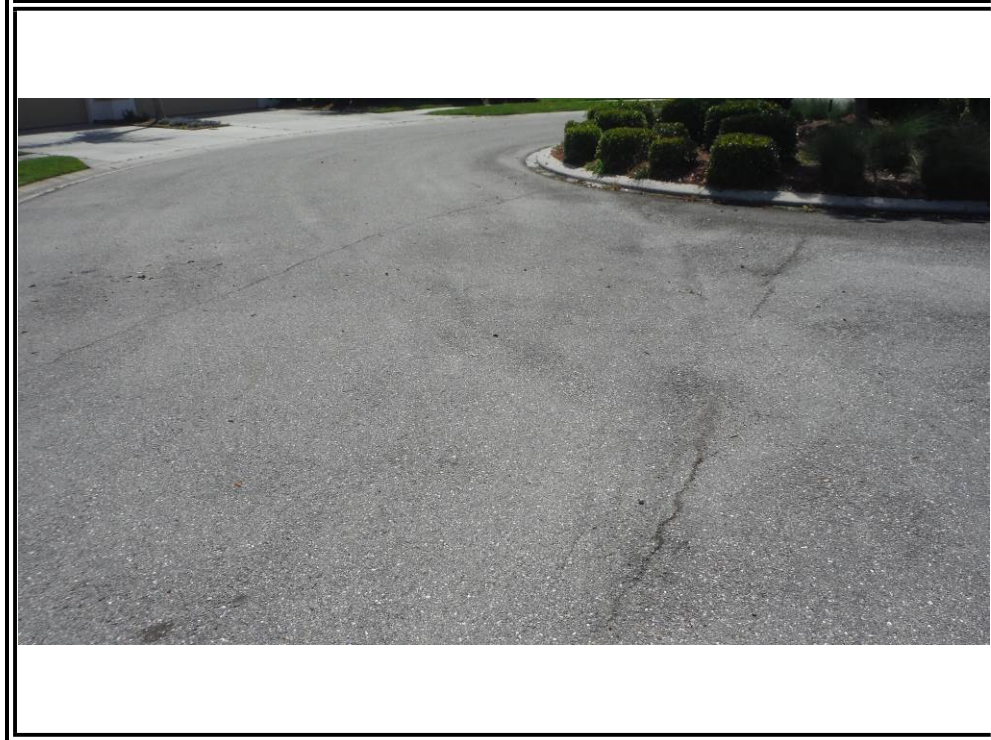
Photo No. 8 Radial Cracking in Cul-De-Sac
