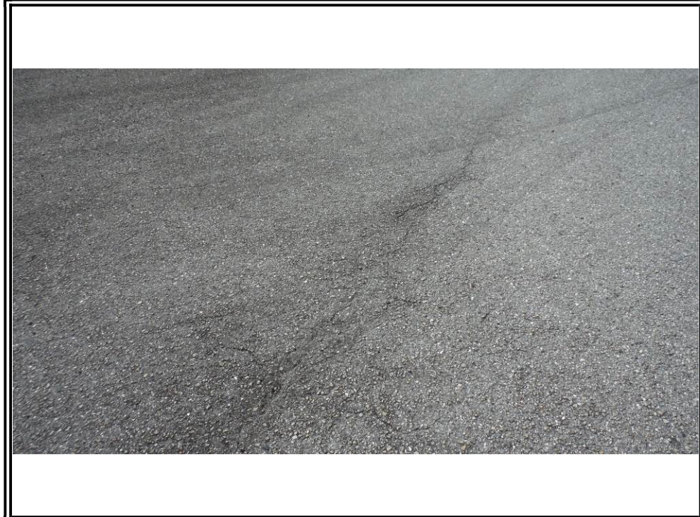
Photo No. 5 Various Minor Cracking
