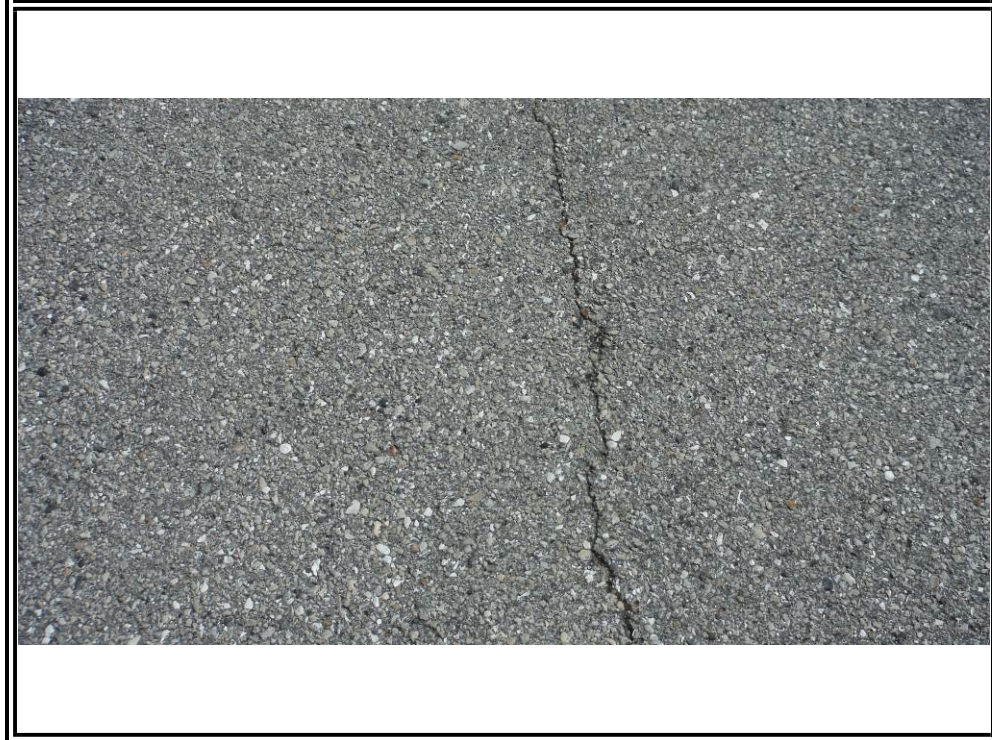
Photo No. 6 Longitudinal Cracking with Seperation
