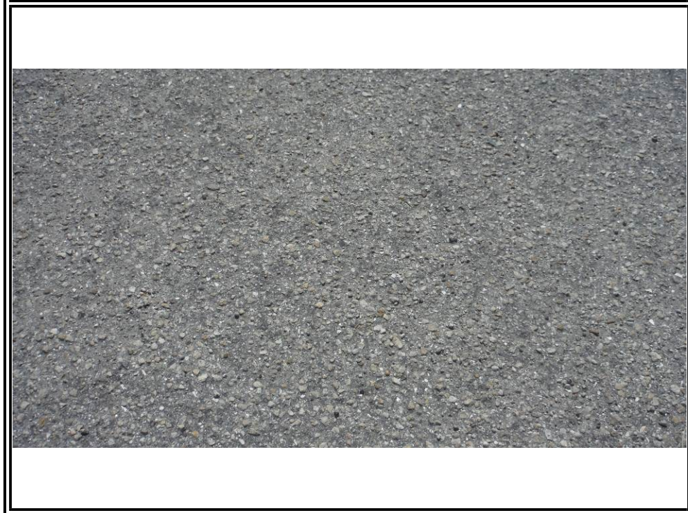
Photo No. 2 Exposed Aggregate in Asphalt Material
