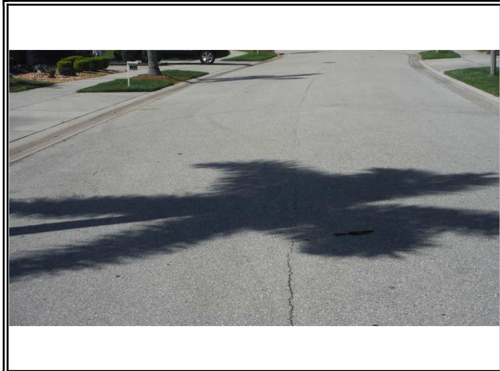
Photo No. 7 Typical Longitudinal Cracking
